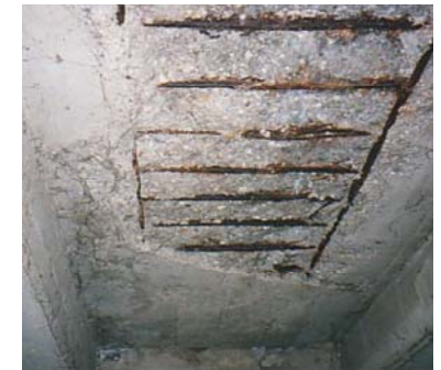
Corrosion of steel in RC bridge deck
